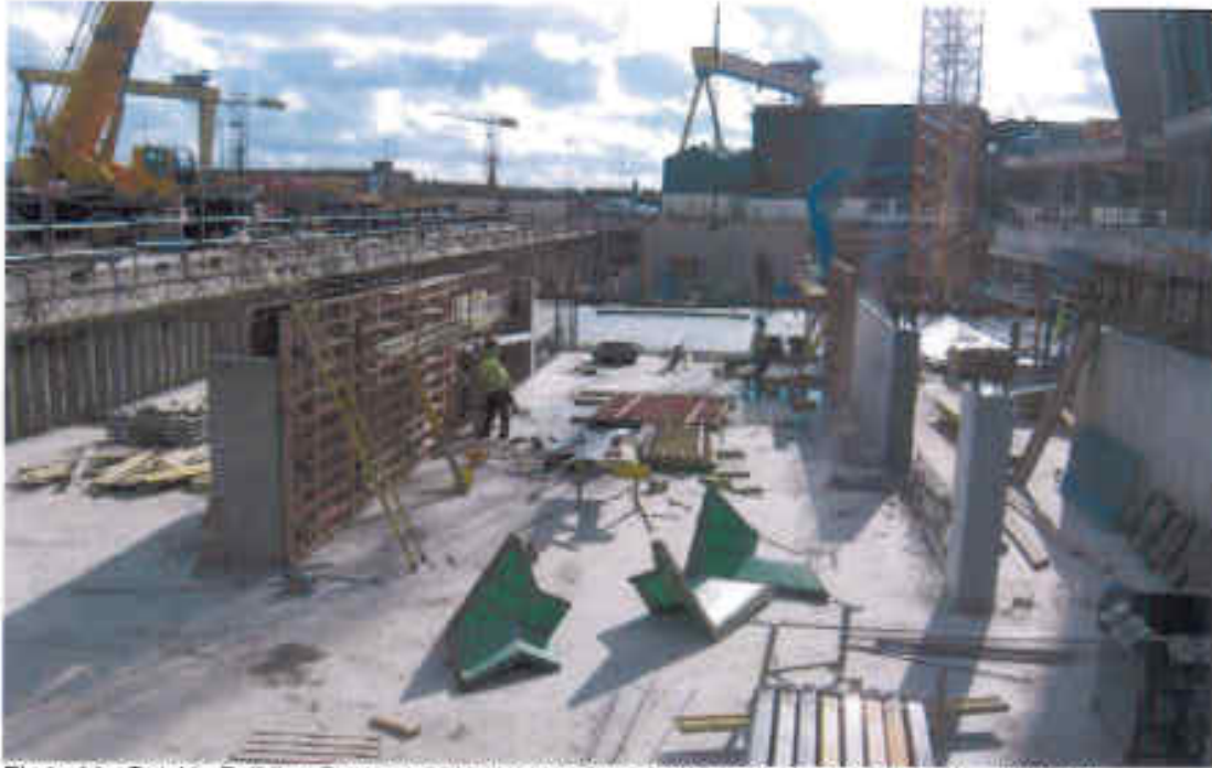
Photo 11: Outside Building Contract (NW Ramp in Construction from -1 to Ground) (as at 8/9/10)
