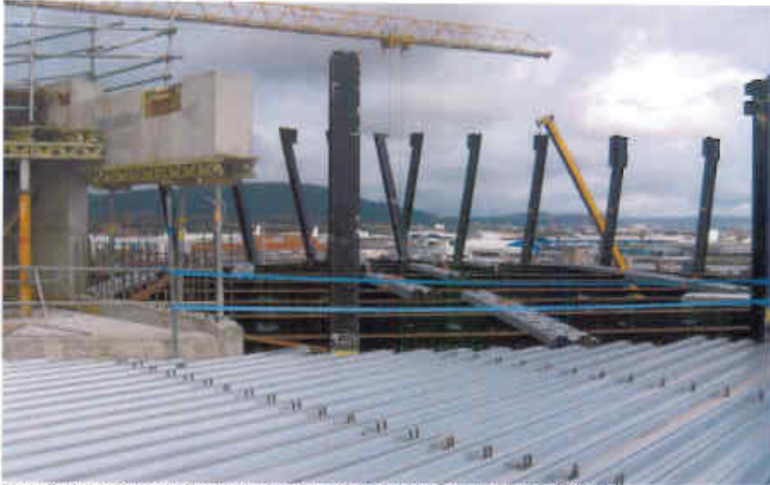
Photo 7: Hull 1 Structural Steel at roof (note: metal decking in foreground) (as at 8/9/10)
